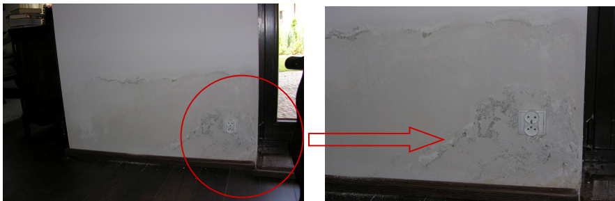
Fig. 2. Exemplary view of damp external walls.
