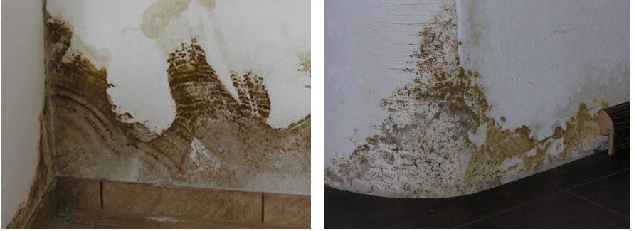
Fig. 3. Exemplary view of damp and infested with rot ground floor walls.
