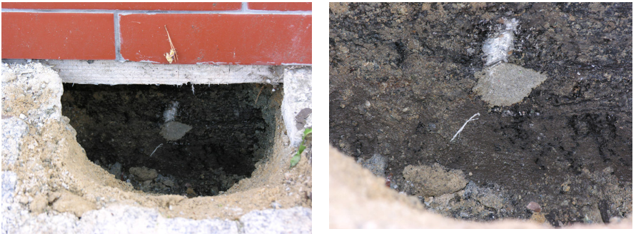
Fig. 4. Test pit revealing damp insulation coating.
