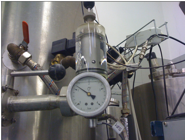
Figure 3: Position of SENSOR2 on the bottom of the carbon dioxide outlet valve assembly. Photo by D. Varner
