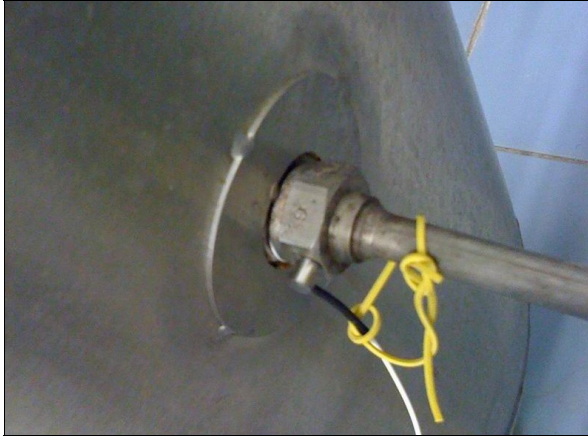
Figure 2: Position of SENSOR1 on the temperature gauge. Photo by D. Varner
