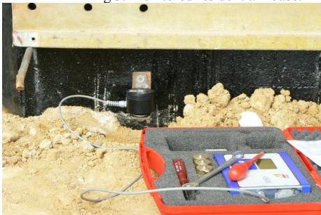
Fig 4. Sensor on the bridge abutment.
