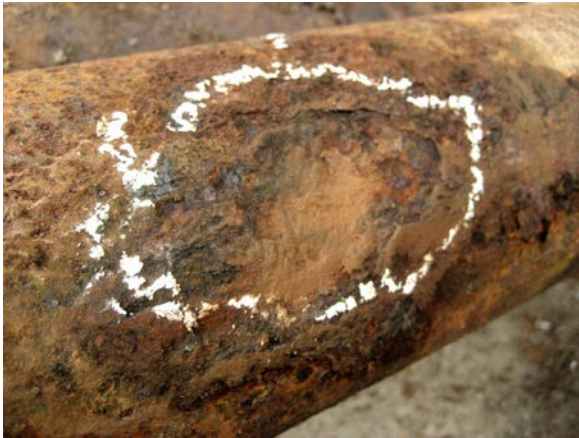
Fig.1 Severe corrosion on pipes.
